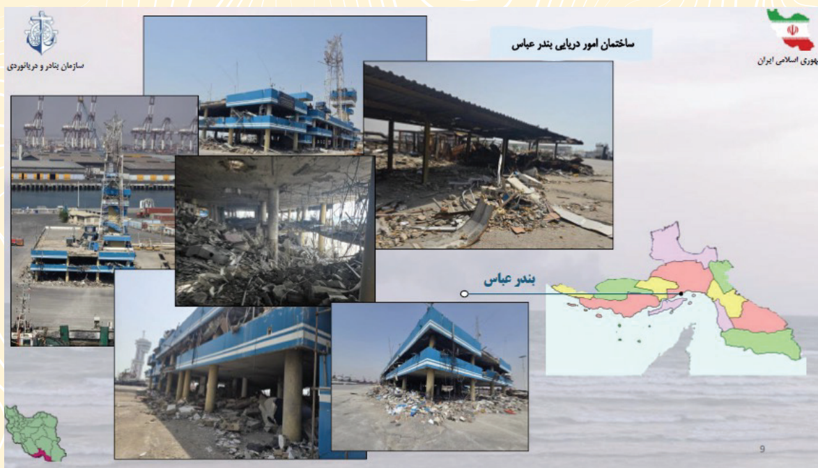
Maritime Affairs Building, Bandar Abbas, following impact and damage
